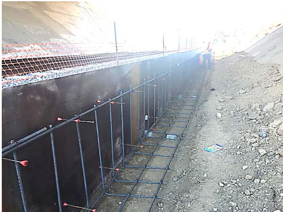
Crews construct the retaining wall north of Rush Creek Place (Novato) that will support the pathway.
