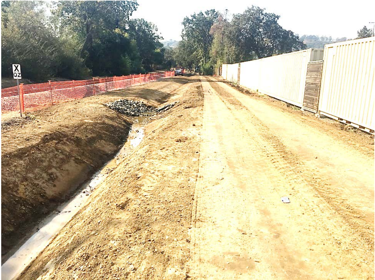
The pathway north of North San Pedro (San Rafael) before crews finished paving.
