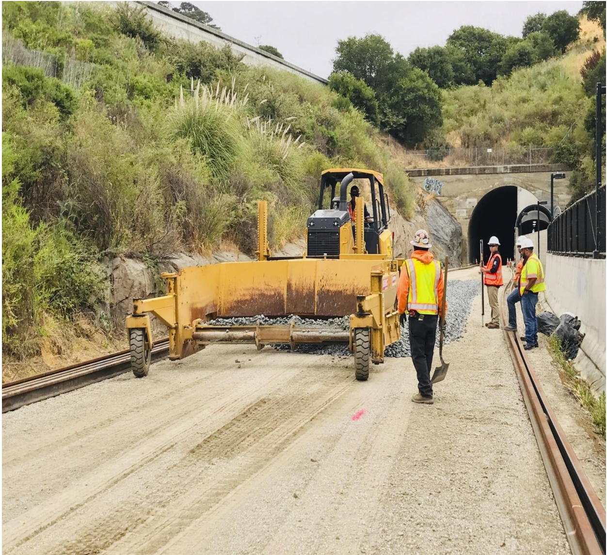
South Cal Park Tunnel to Station placing the gravel ballast for the track
